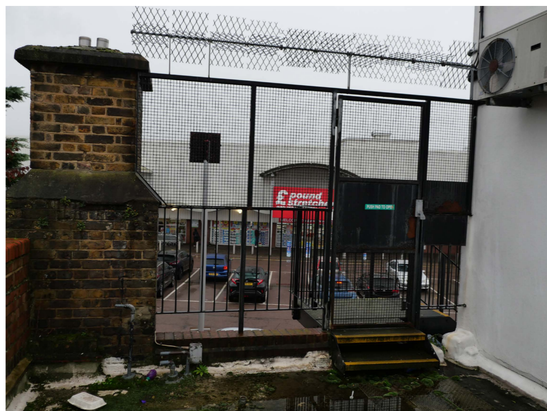
1st fl. roof terrace to east showing security screen on fire escape route with plant room chimney
